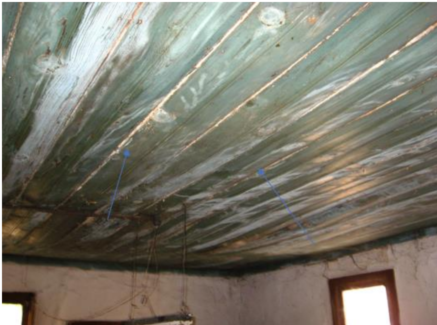
Figure 3. Nevzat Akay House of bending caused by mechanical effect on the ceiling covering.
