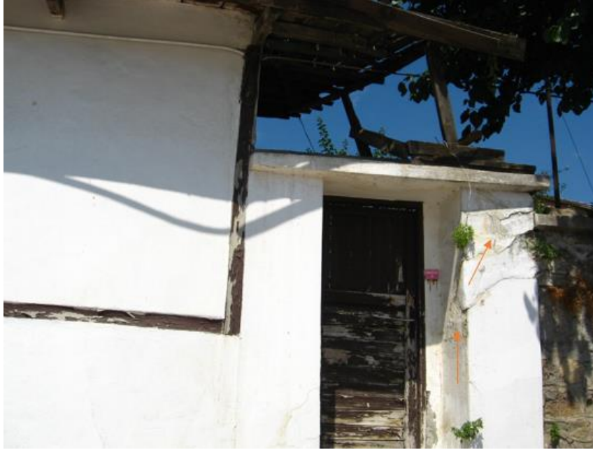
Figure 8. Nevzat Akay House of deteriorations caused by the effect of heat on the exterior of the sturcture.
