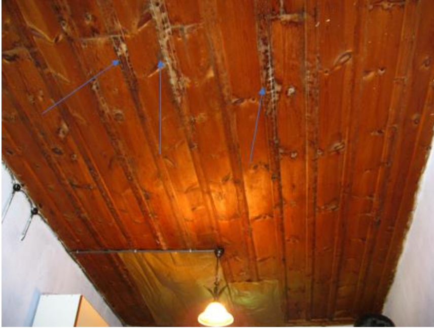
Figure 2. Ayşe Sezgin House of bending caused by mechanical effect on the ceiling covering.
