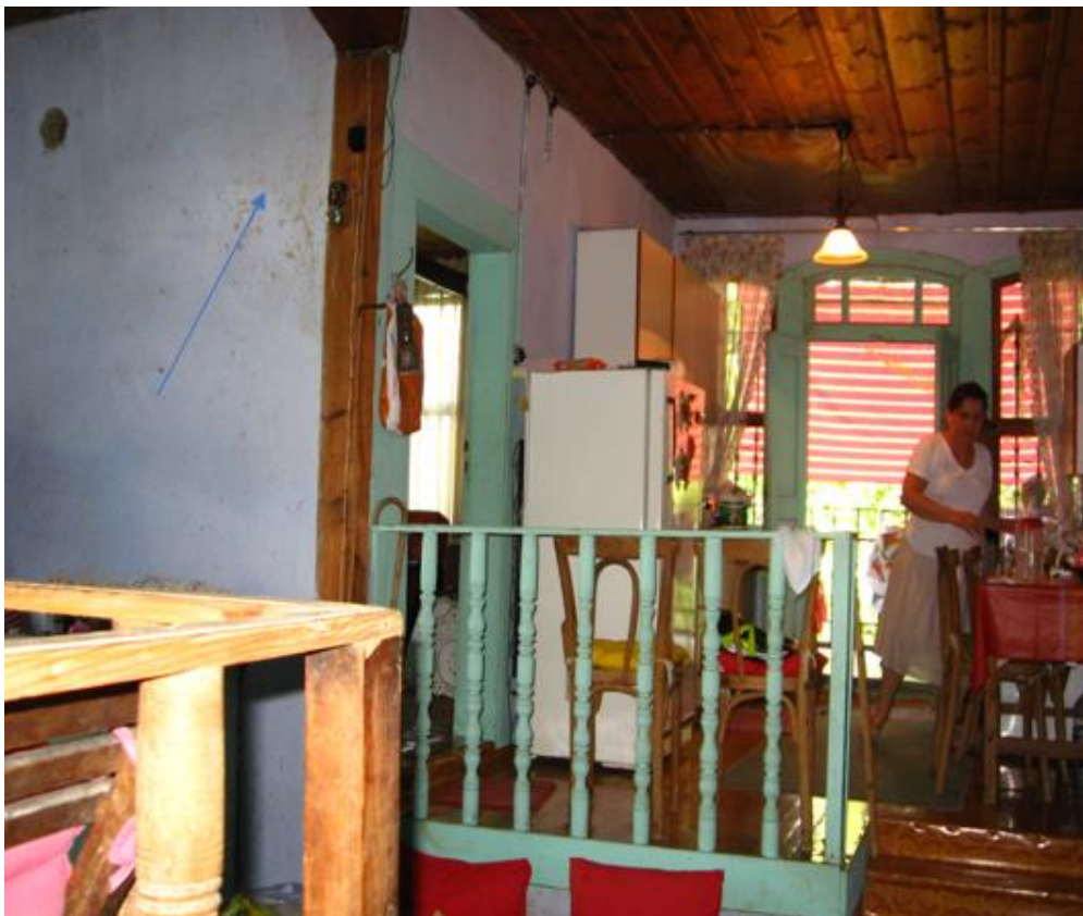
Figure 11. Ayşe Sezgin House of deterioration of the wall surface due to water and moisture.
